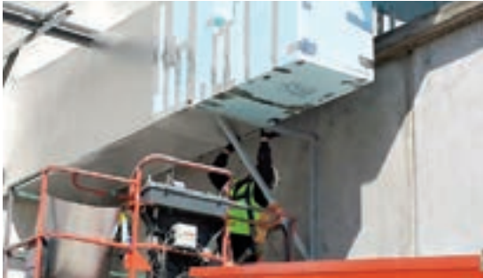
TRADING UP Mike Bradley of Iowa Insulation installs a protective aluminum jacket over 2-in.-thick Styrofoam insulation on an outdoor duct at a feed mill in Hedrick, Iowa.
