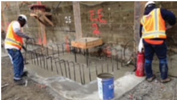
Pile caps and rebars for the Sacramento Kings new arena were coated and cured with Xypex in one day.
