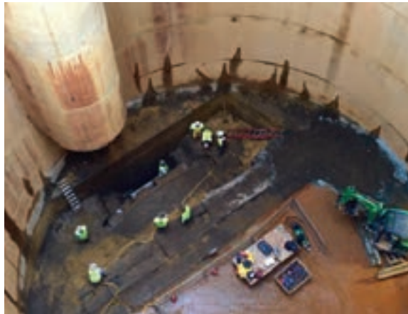
Lady Bird receives cutterhead maintenance at the Poplar Point, D.C. junction/drop shaft in early April.
