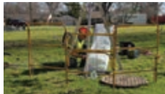
For a sewer line rehabilitation, Michels installed a pre-liner through a manhole in a residential area.
