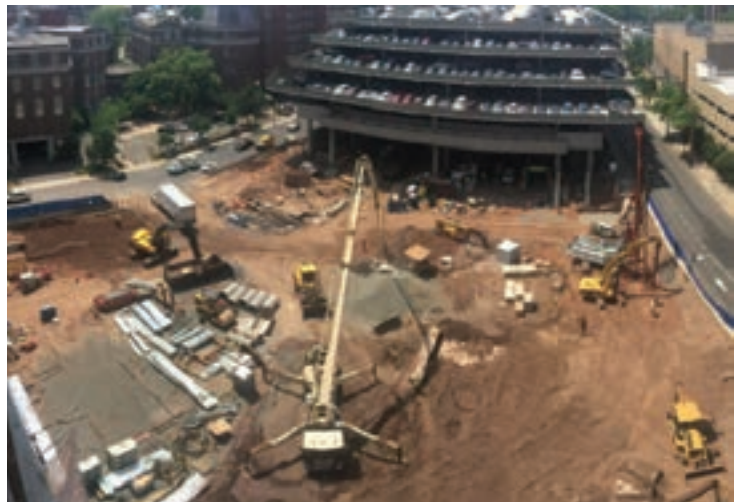
Geopier ground improvement solutions support a 12-story office building and parking garage in New Haven, Conn.
