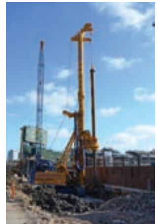
Case Foundation installed 69 belled caissons to support new outfield bleachers at historic Wrigley Field.
