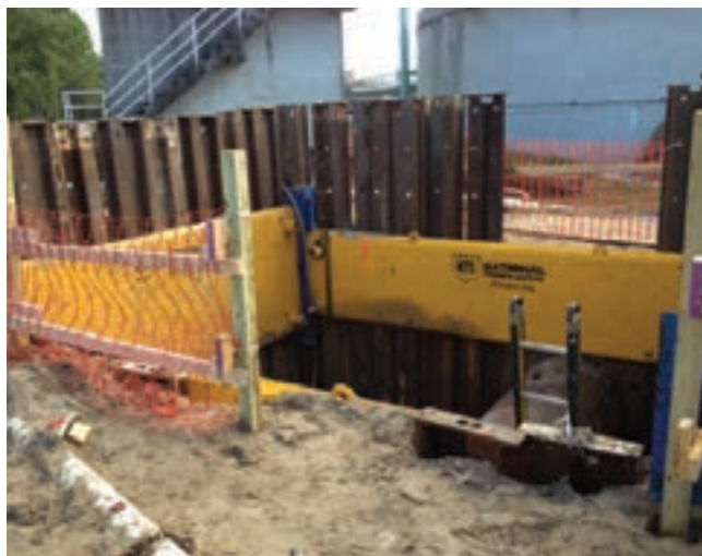
Selecting a steel sheeting guide frame system for unstable soils that also protects crossing utility lines was key to this project's success.
